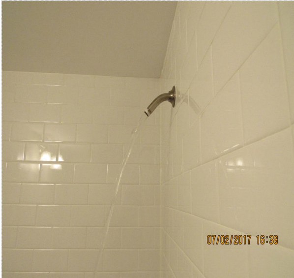
IMG_6420.JPG Missing shower head.
